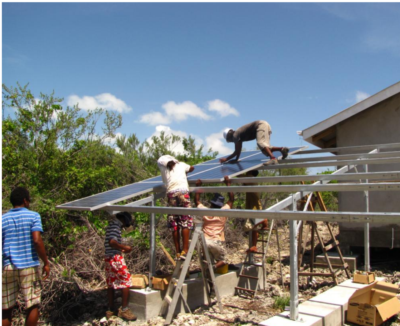
SIF staff on Aldabra assembling solar modules on mounting frame © Christina Quanz (March 2012)
